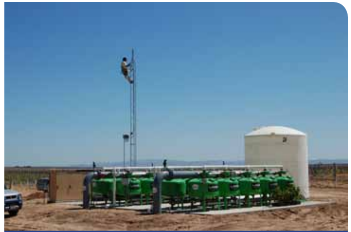
A Tesco Controls communications engineer installing an antenna for wireless Ethernet communications.
