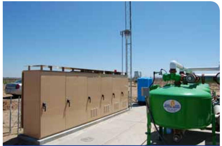
Tesco Controls' motor control center in the freshly planted vineyard. Note the sun shields on top and back. The sun shields provide a 15 degree reduction in temperature on the enclosure.
